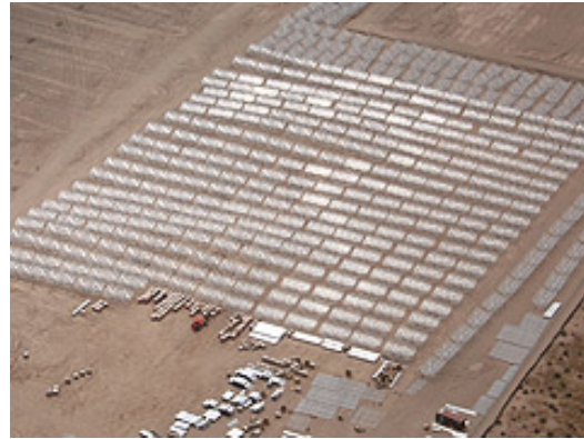
Assembly of the parabolic-trough system components is underway for the 64-Megawatt Nevada plant, which will generate enough electricity to power about 11,000 homes. Credit: Solargenix
